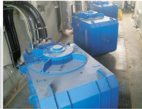
1200 hp influent pump motors
