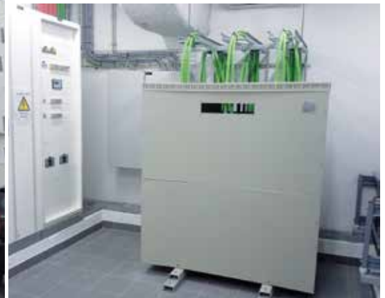
From left to right: The low voltage security panel with switch gear and Bender devices and on the right side the 630 kVA isolation transformer 400/400 V.
