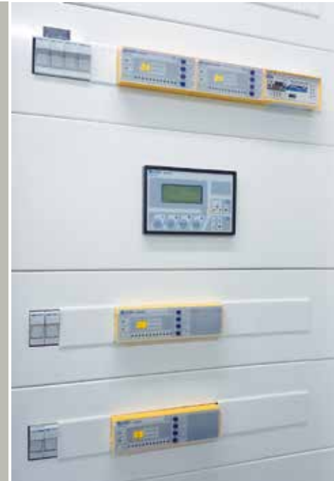
Low voltage security panel with switch gear and Bender devices
